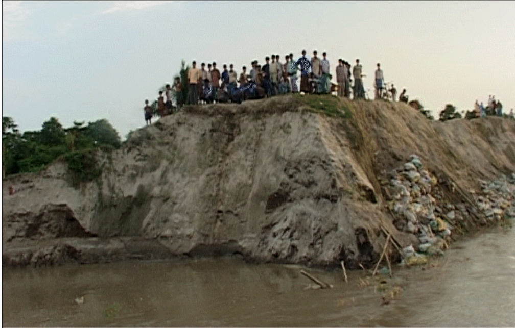
Plate-4: The breached embankment near Panchanandapur. Here the encroaching river threatens to outflank the Farakka Barrage.
