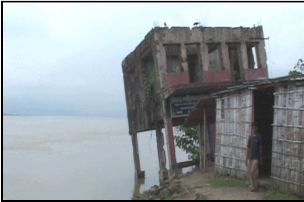
Plate-8: The deserted house leans towards the Padma at Jalangi.
